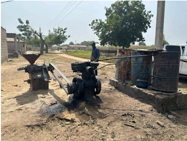
FIGURE 3: A diesel-powered rice mill in Saachi Nku community, Niger state. Photo taken by the author in November 2023.
